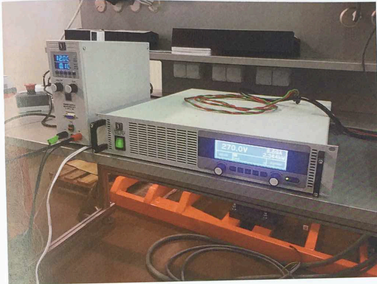
DC supply blocks
